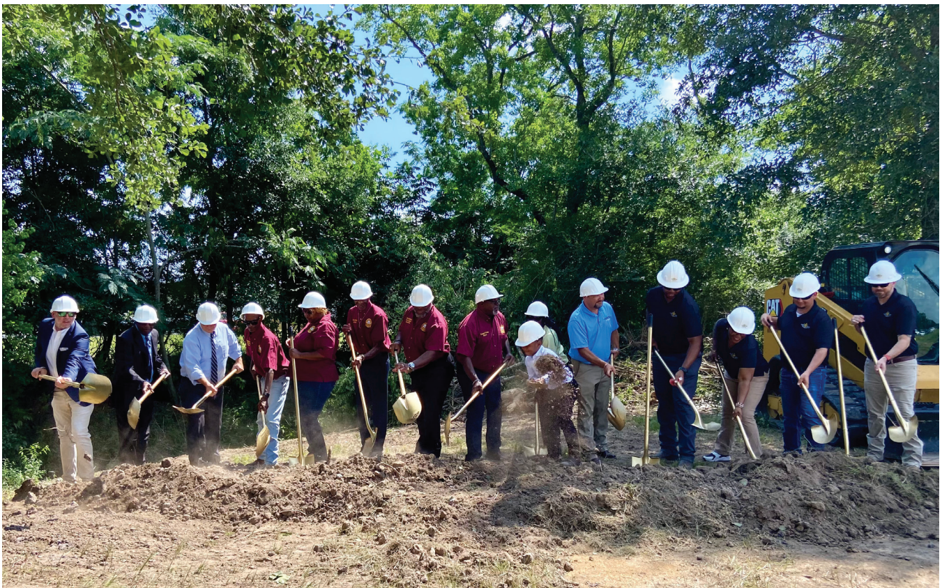
The Bayou Lacombe Channel Improvements Project Groundbreaking, June 2024. This project will benefit watershed regions 2 and 5.
